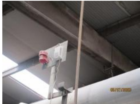
Siren and Gas Detector.jpg
