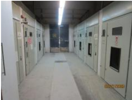
Main Electricity Panel.jpg
