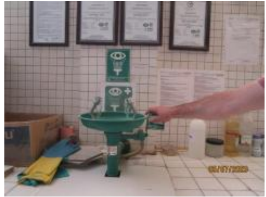
Eye wash station.jpg
